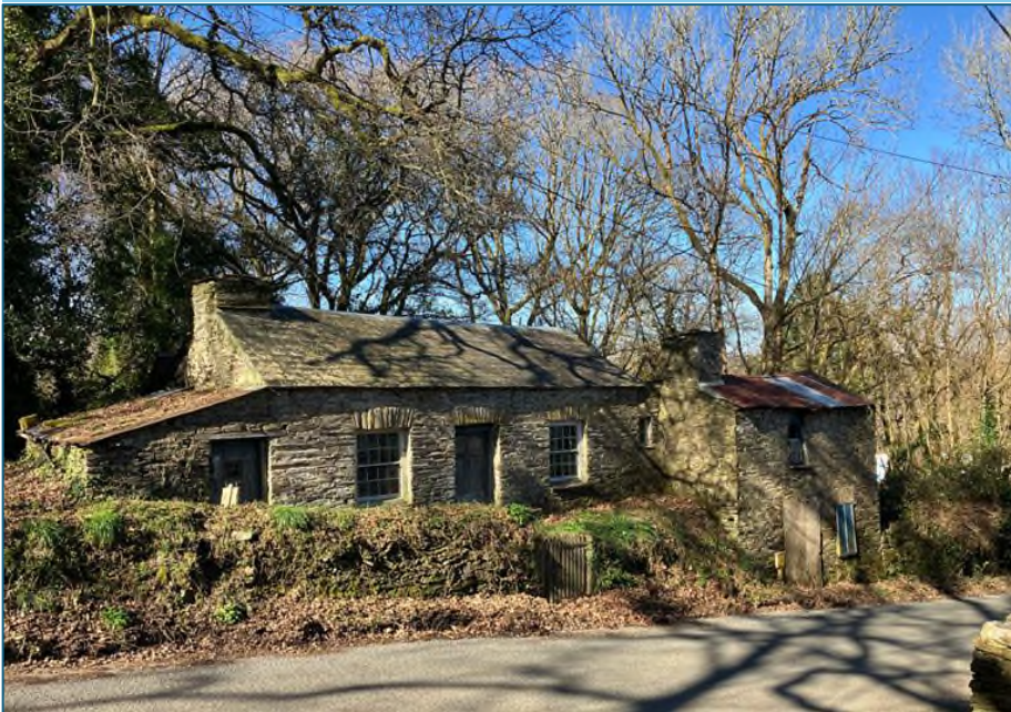
Photo: Declining Grade II Listed Buildings, Lucket Hill.
